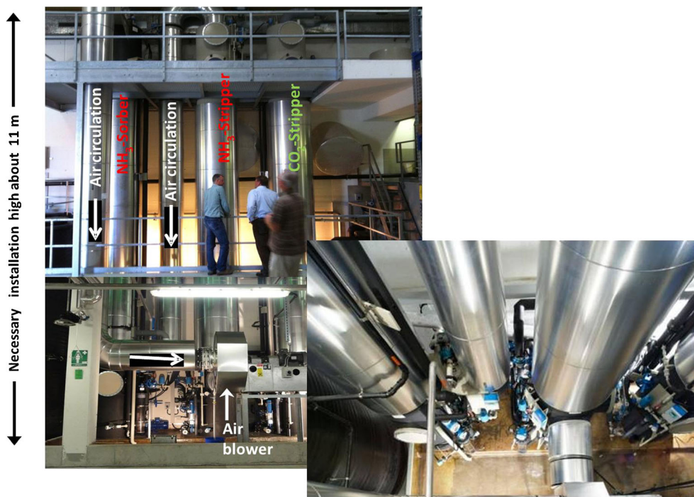
Fig. 2 Full scale air stripping plant at WWTP Klotten/Opfikon
