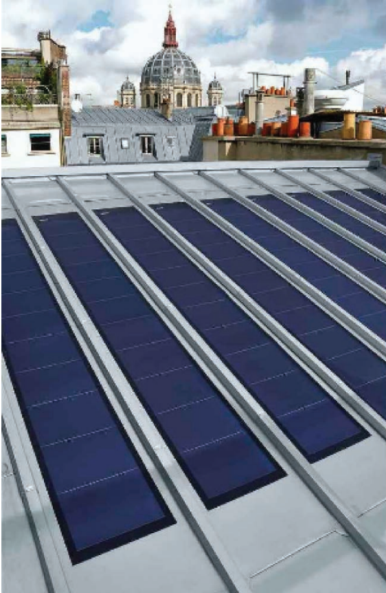
Fig. 13: PV applied on zinc standing seam panels
