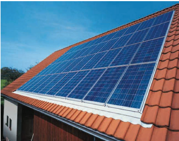
Fig. 19: Framed in-roof system: less homogenous appeal due to the contrast of the aluminium frame and the PV panels.
