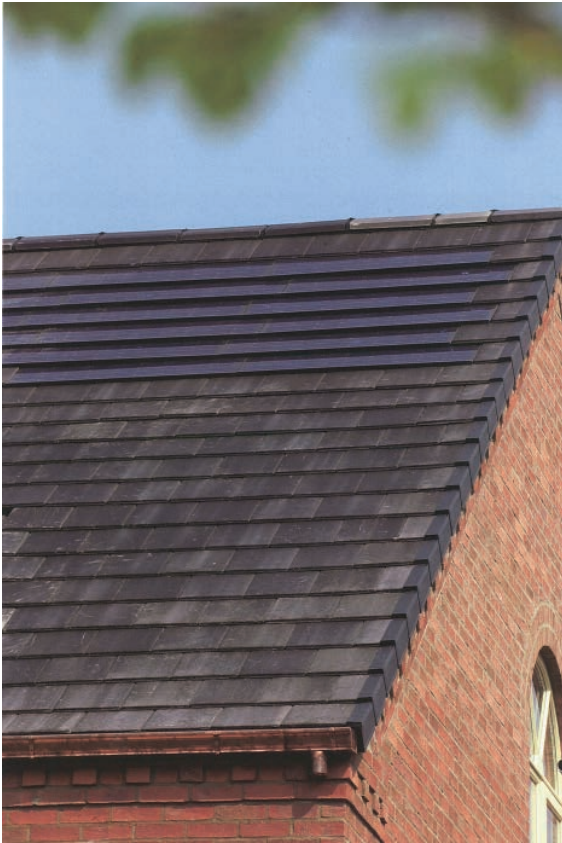
Fig. 26: Residential estate, Allington (England): solar shingles seamlessly inserted replacing conventional tiles (Surface: 9, 6 m 2 , Energy output: 1 kWp; System provider: Solar Century, 2003; Source: Hermannsdörfer/Rüb 2005)
