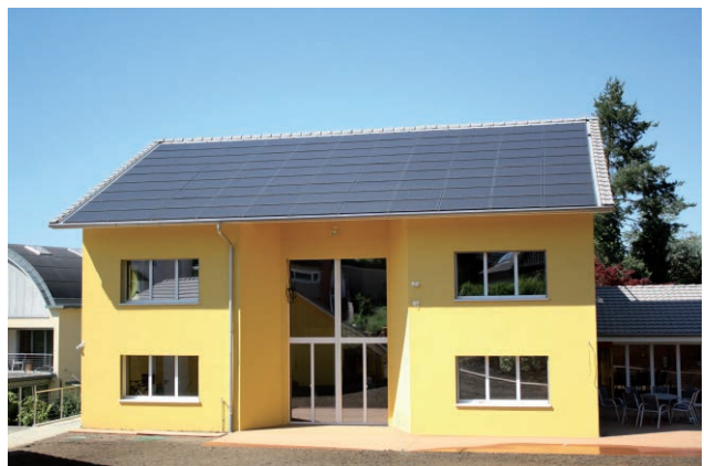
Fig. 21: Full-roof installation with c-Si panels (System provider: 3-S Photovoltaics, Meyer & Burger Group)
