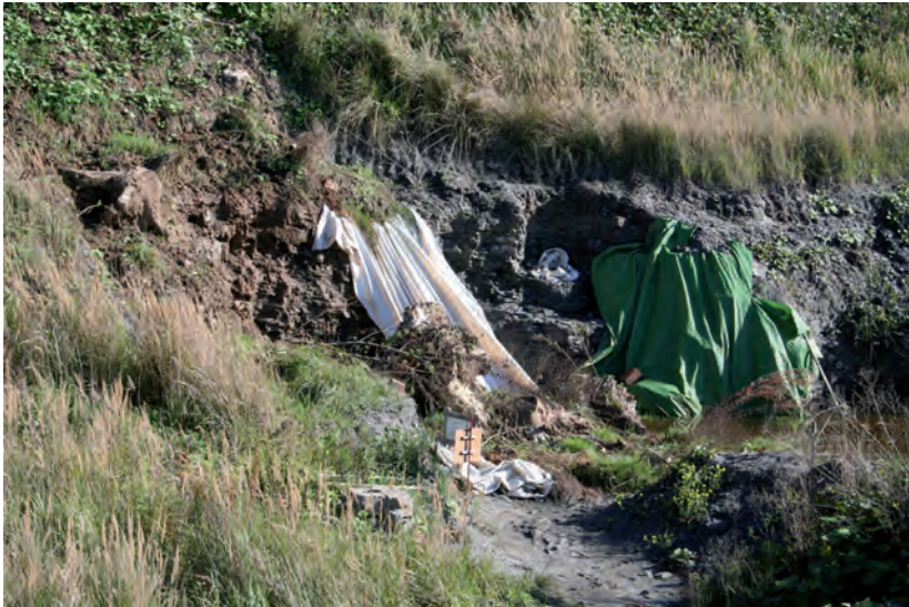
Figure 6: One of the landslides that terminated the excavation in autumn 2008. The grey material represents the Fish Shale.
