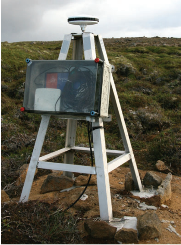
Figure 2. Example of a set up for the continuous GPS stations in North Iceland. The stainless-steel quadripod of the station SAVI is drilled and cemented into the ground. The box protects the GPS receiver and the wireless LAN antenna, which is used for data transmission to an Internet access in 6 km aerial distance.
