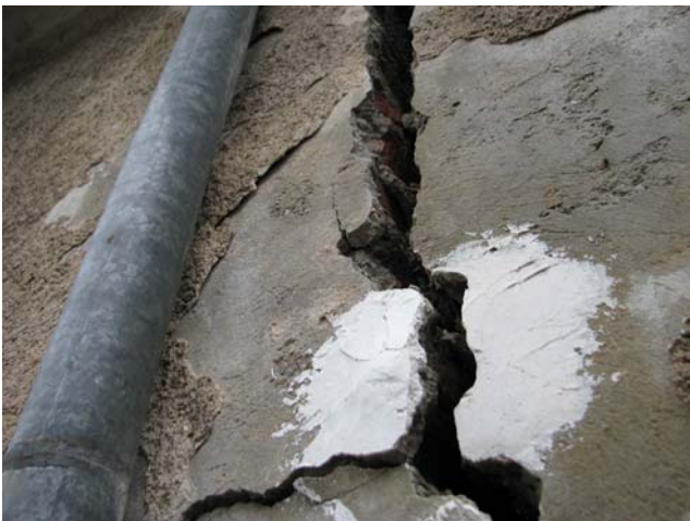
Fig. 2 One of the largest cracks (rainwater gutter for size comparison) in the city centre of Staufen
